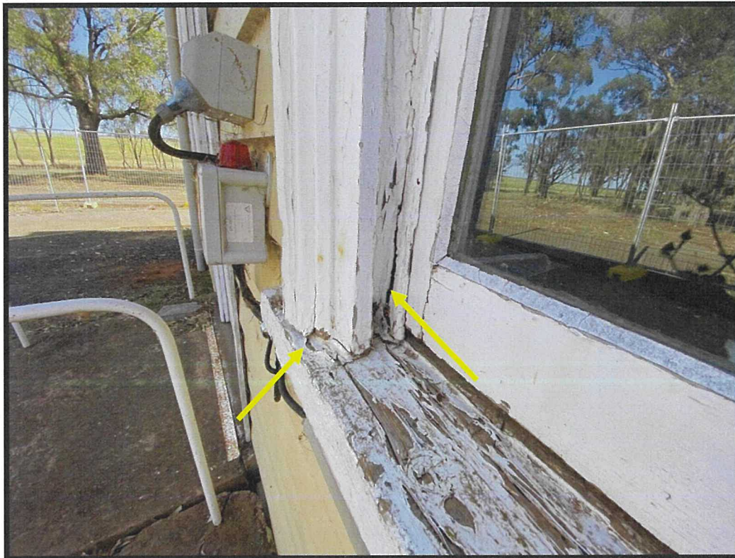
Photograph 5 – Typical dilapidation to the window frames along the building perimeter. Note the timber splitting and sealing dilapidation.
