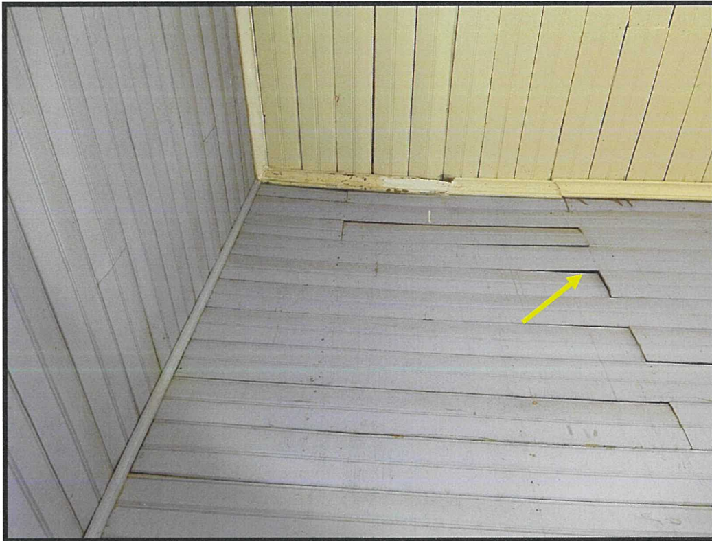
Photograph 13 – Typical detachment/misalignment of the internal lining boards of the wall on the east side of the stage.
