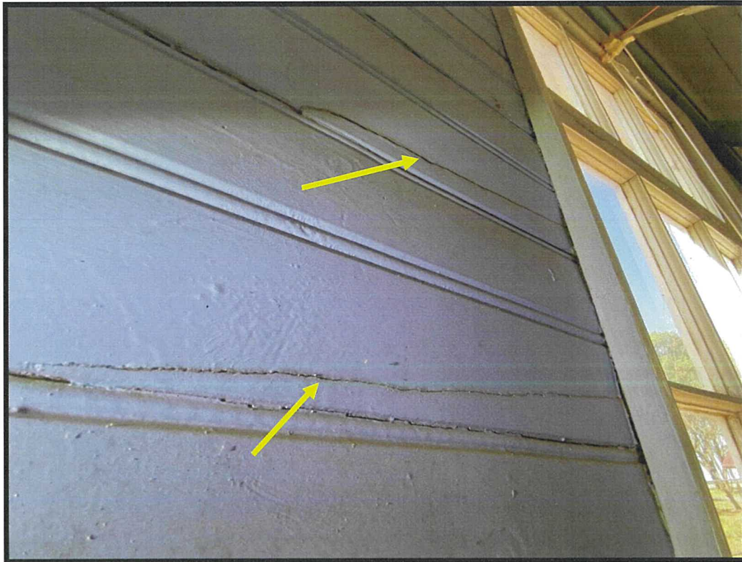
Photograph 15 – Typical pre-existing splitting to the internal lining boards of the northern wall.
