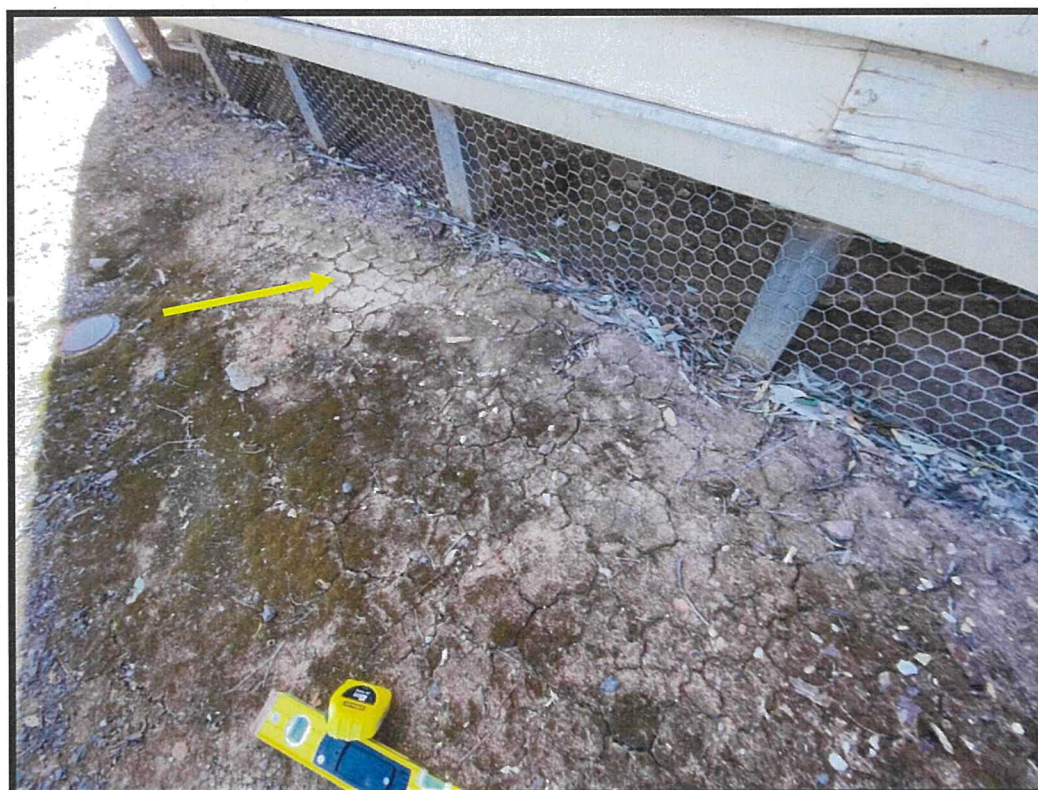
Photograph 6 – Typical cracked dried soil surface adjacent to the building perimeter.
