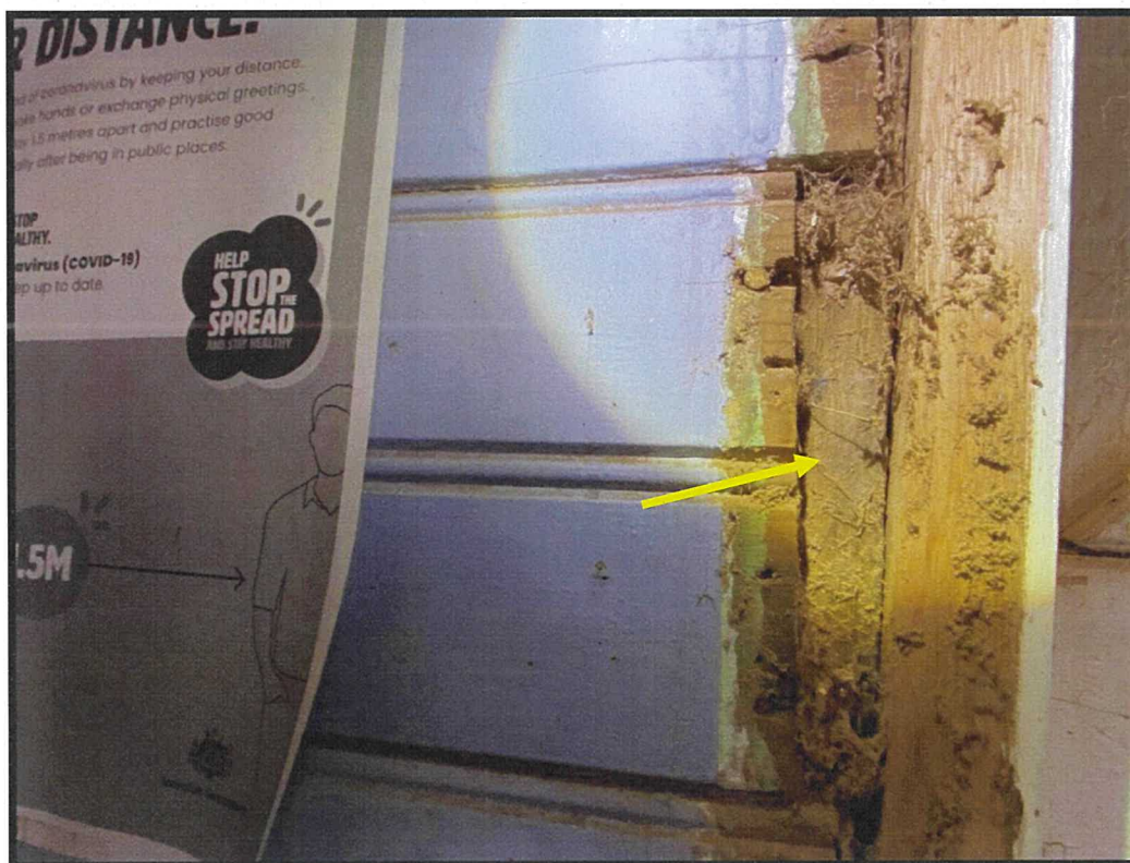
Photograph 12 – Exposed timber stud adjacent to the door frame of the on western wall of the building.
