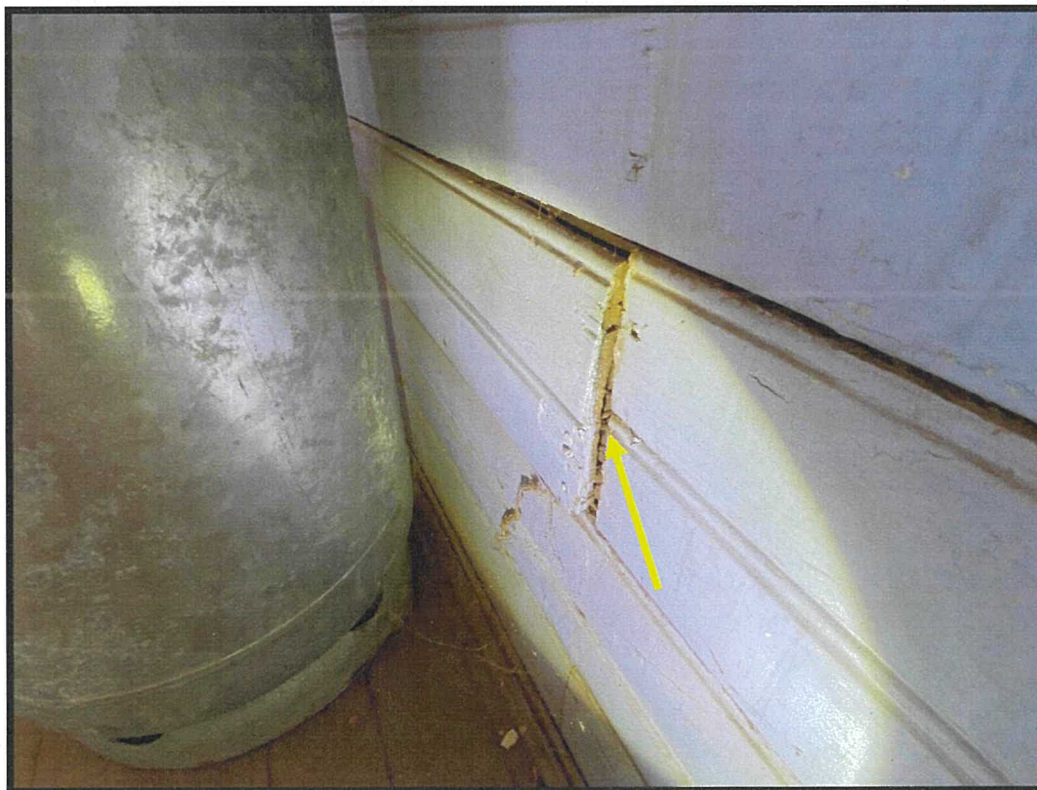
Photograph 14 – Typical detachment/misalignment of the internal lining boards of the northern wall.
