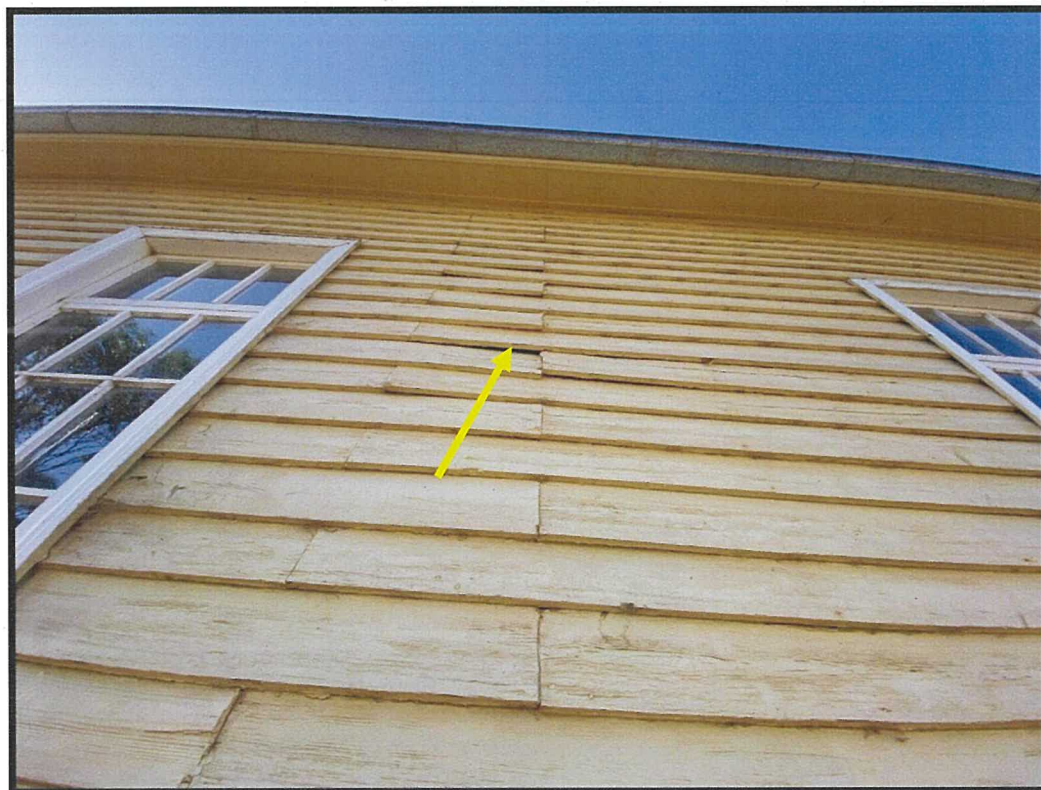
Photograph 4 – Typical splitting, detachment/misalignment to the weatherboard cladding.
