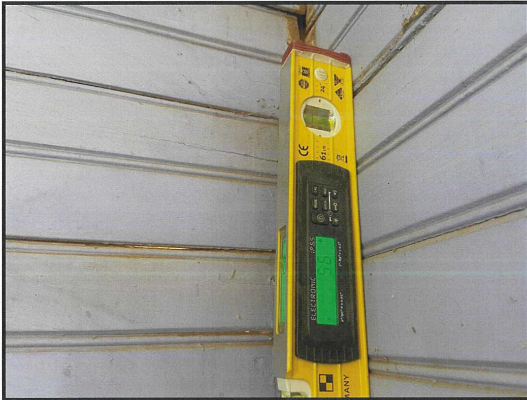
Photograph 9 – The west end of the building is leaning towards the north by 3.2° (56mm/m).
