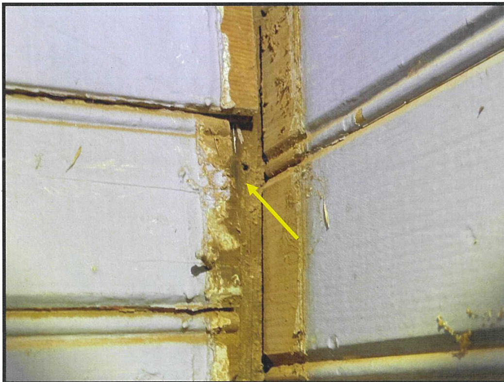
Photograph 10 – Minor staining to the exposed timber stud at the north end of the western wall of the building.
