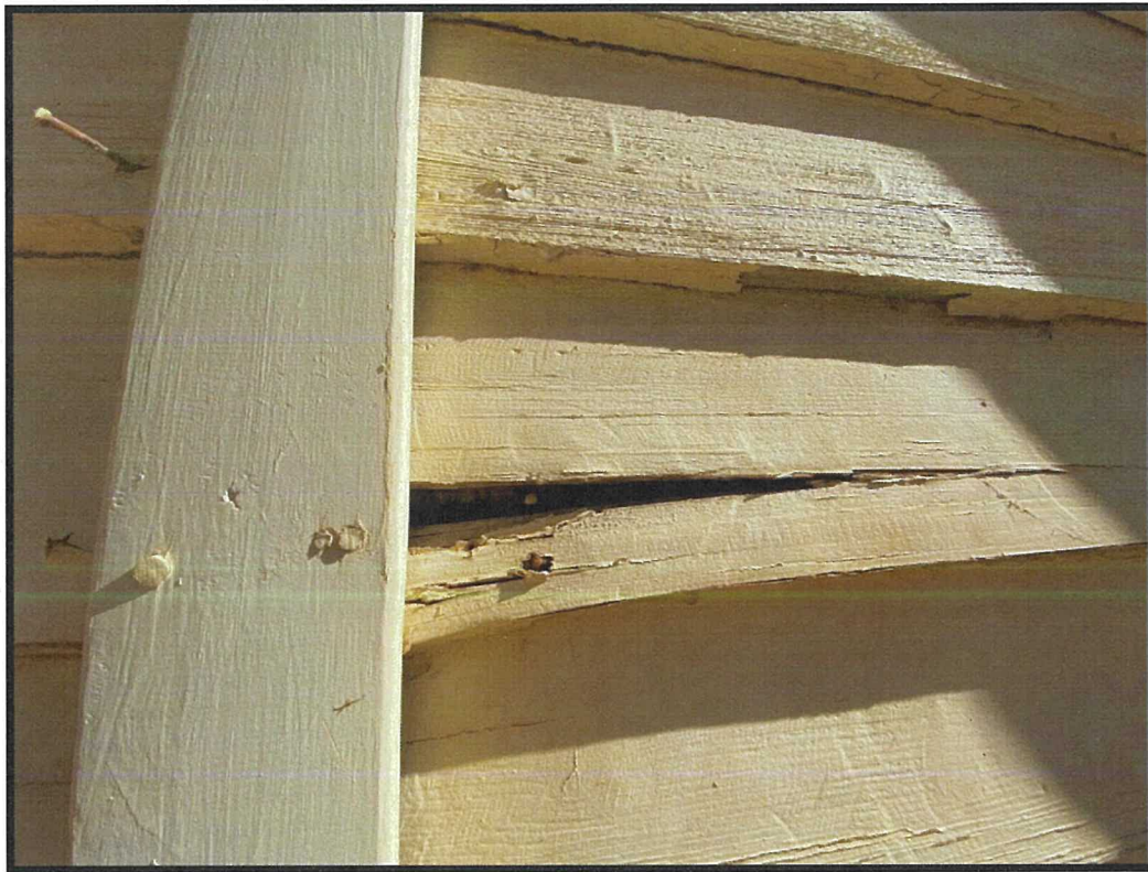
Photograph 3 – Timber splitting to the weatherboard cladding.
