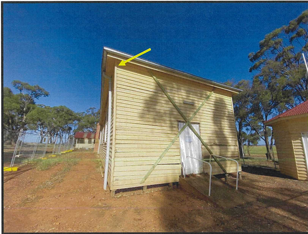
Photograph 1 – The west end of the building is leaning towards the west by 3.2^\circ (56mm/m). Temporary bracing has been installed as part of the make safe works. Note the unsealed ground immediately adjacent to the building perimeter.
