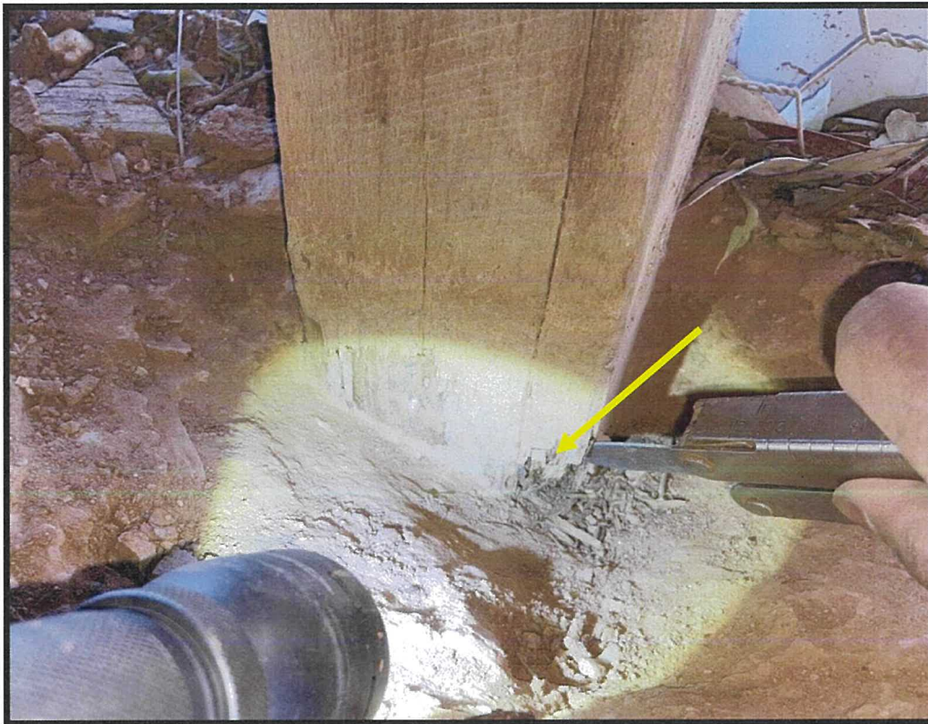
Photograph 19 – Decay to a perimeter timber stump.
