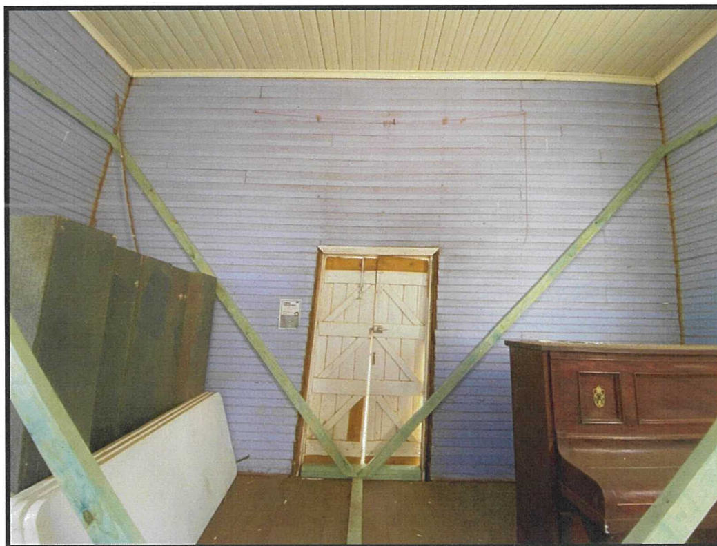
Photograph 8 – Deformation of the western wall.
