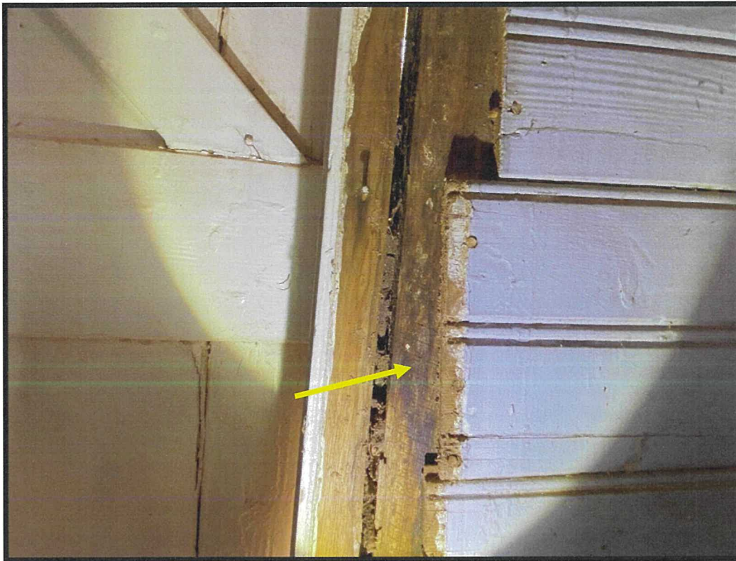
Photograph 11 – Staining to the exposed timber stud adjacent to the door frame of the on western wall of the building.
