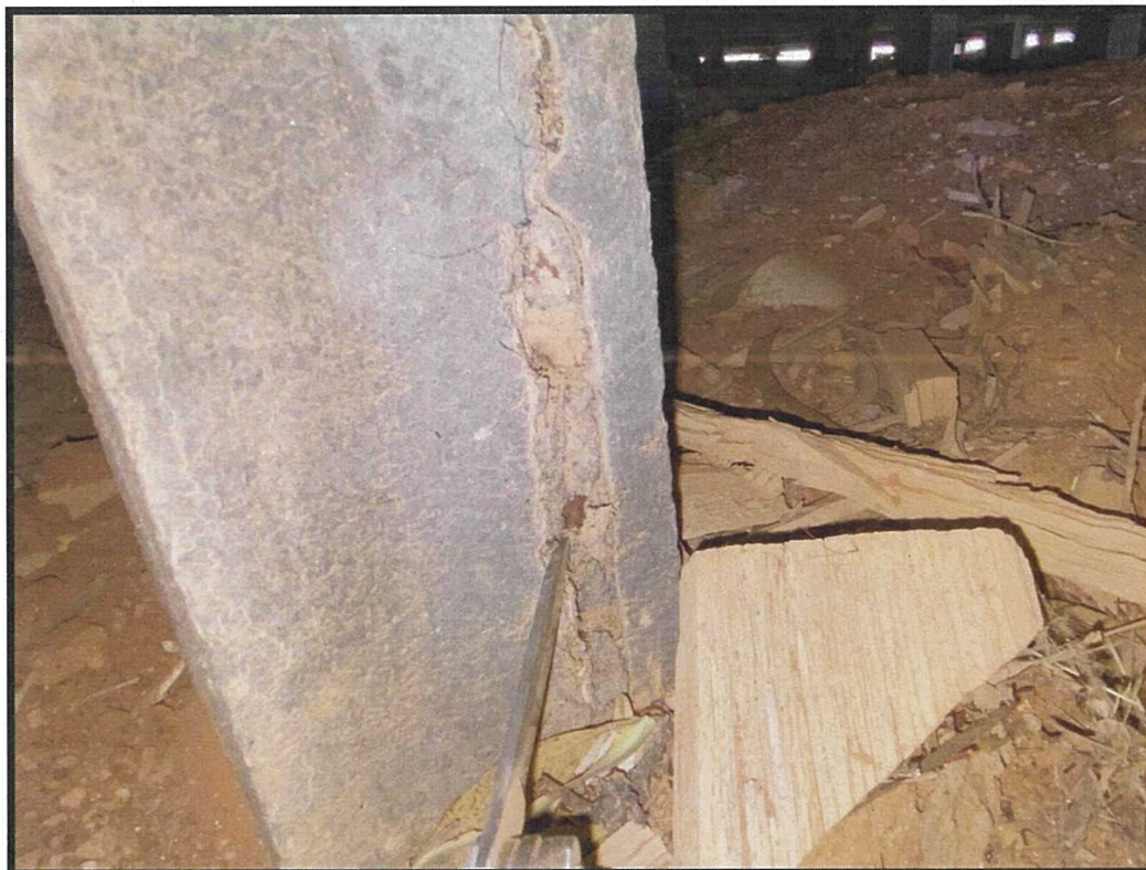
Photograph 20 – Minor decay to an internal timber stump.
