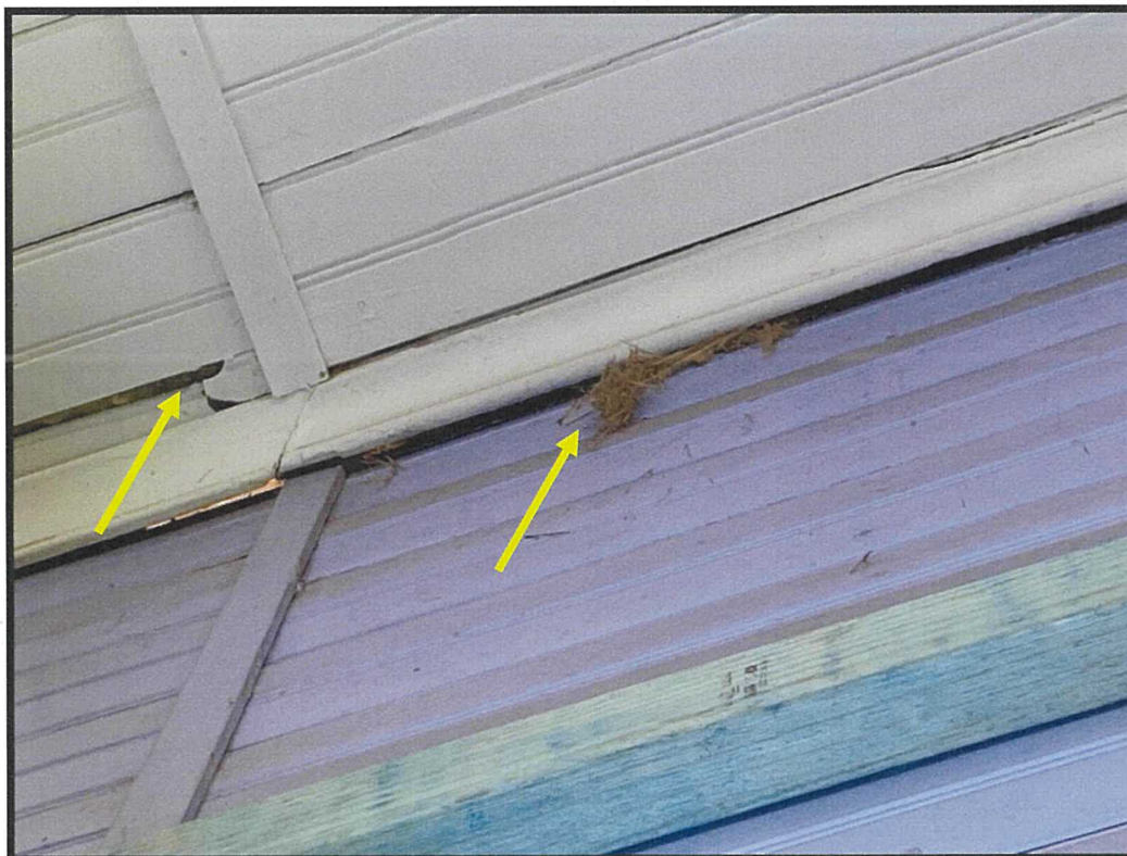
Photograph 16 – Detachment of the timber cornice and cracking to the ceiling boards on the north end of the hall.
