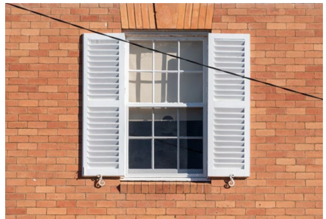
Figure 23: A building that has retained its original, unpainted brick finish, reflecting its intended appearance.
